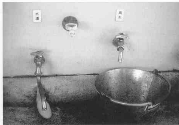
Fig. 7: ▶▶ MIYAKE ISLAND ELEMENTARY SCHOOL: SUPPLY OF TAP WATER (LEFT) AND RAIN- WATER (RIGHT)
