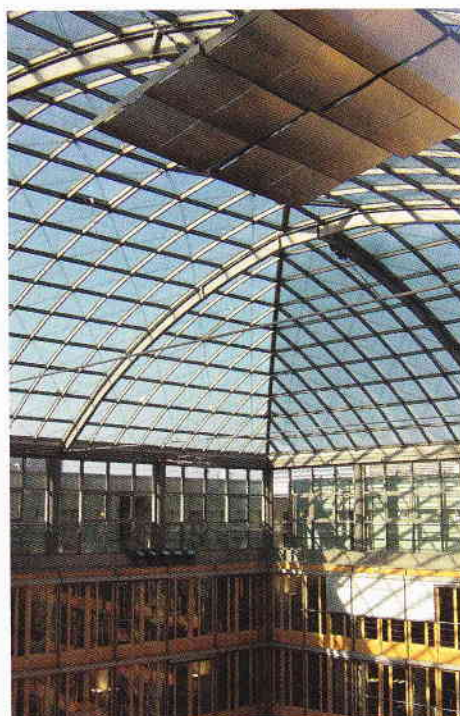
Figure 2: Glass roof over inner courtyard as collecting point for rainwater; the wooden facade of the inner courtyard is protected against fire by a facade rainwater sprinkler system (Photo: Klaus W. König).
