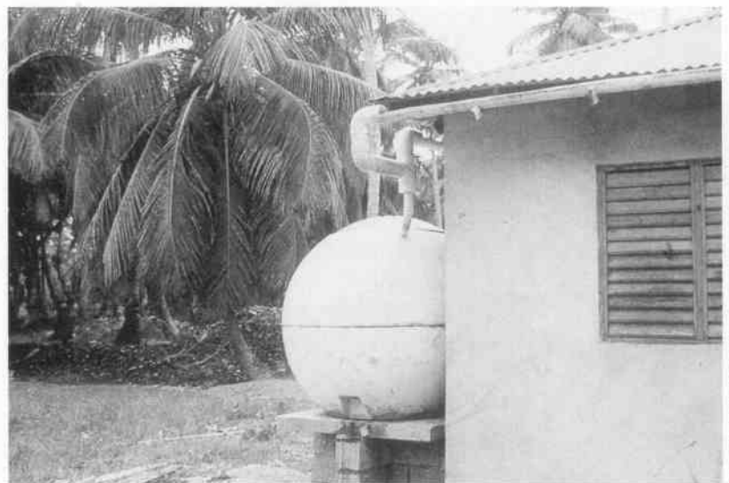
Fig. 3 IN THE DOMINICAN REPUBLIC RAIN WATER SUBSTITUTES DRINKING WATER AND IS DIRECTLY LED TO THE KITCHEN WITHOUT THE HELP OF A PUMP
