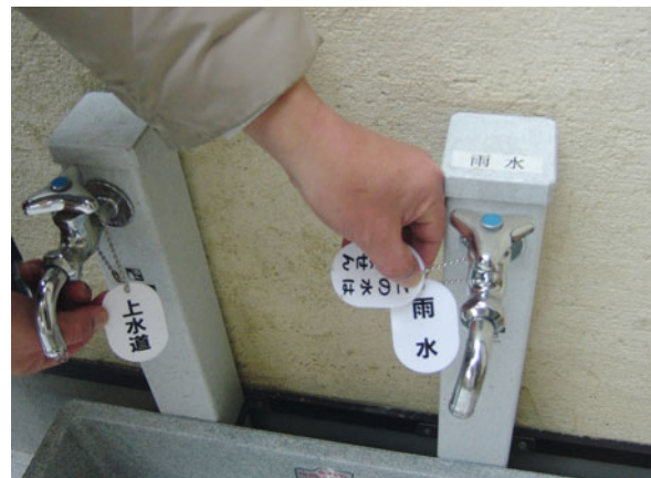
Fig. 4. External washbowl with dual connection drinking water (left) and rainwater. Photo: König
